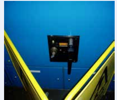
DA 4000 ACB: Access Restricted Due to Nuisance Tripping
